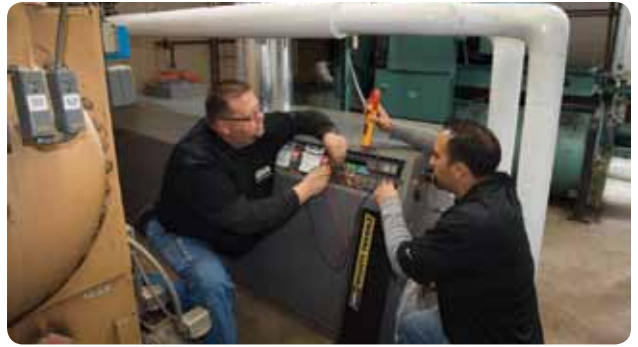
Gary Holbrook and Eric Tafoya service a Laars boiler at Summit Apartments.
