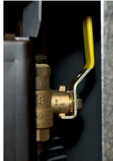
Fig. B15-2 - Gas shutoff valve (typical)
