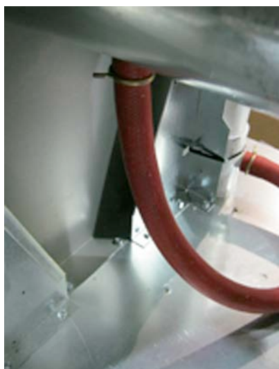
Fig. C5-14 - Drain hose connected under the heat exchanger
