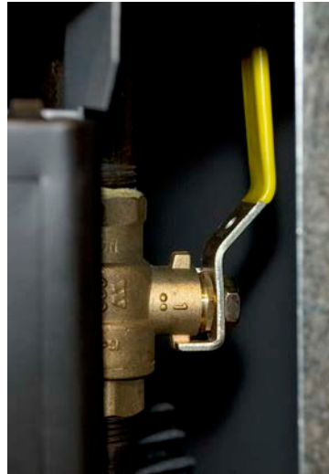
Fig. B11-1 - Gas shutoff valve (typical)
