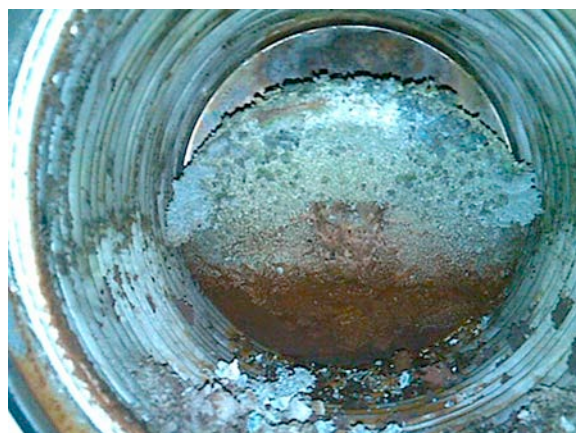
Fig. C5-13 - Very dirty heat exchanger
