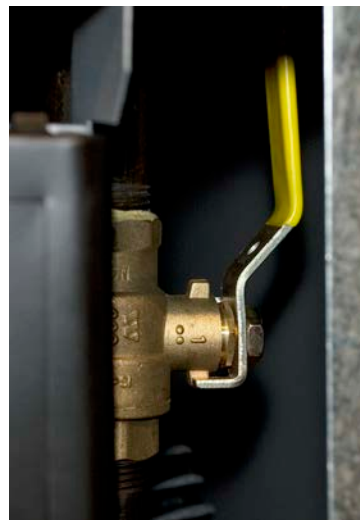
Fig. B23-1 - Gas shutoff valve (typical)
