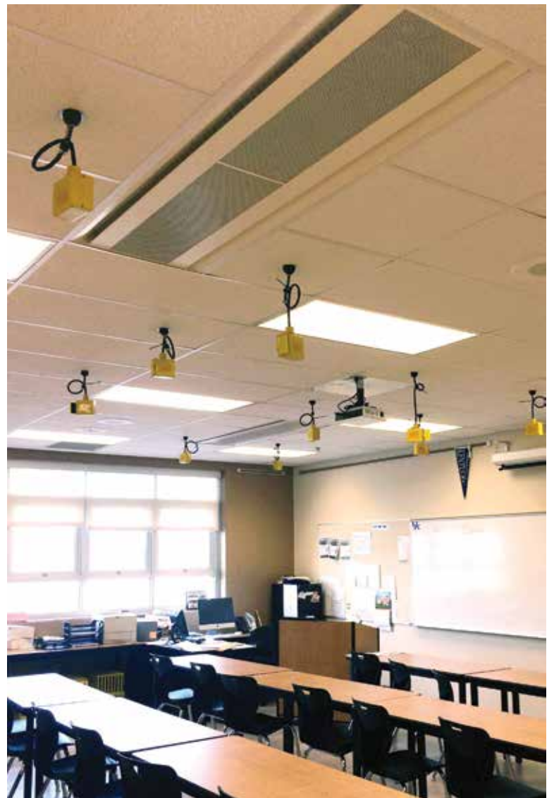
Chilled beams don’t require filters or any moving parts, which reduces the number of maintenance-related classroom interruptions.
