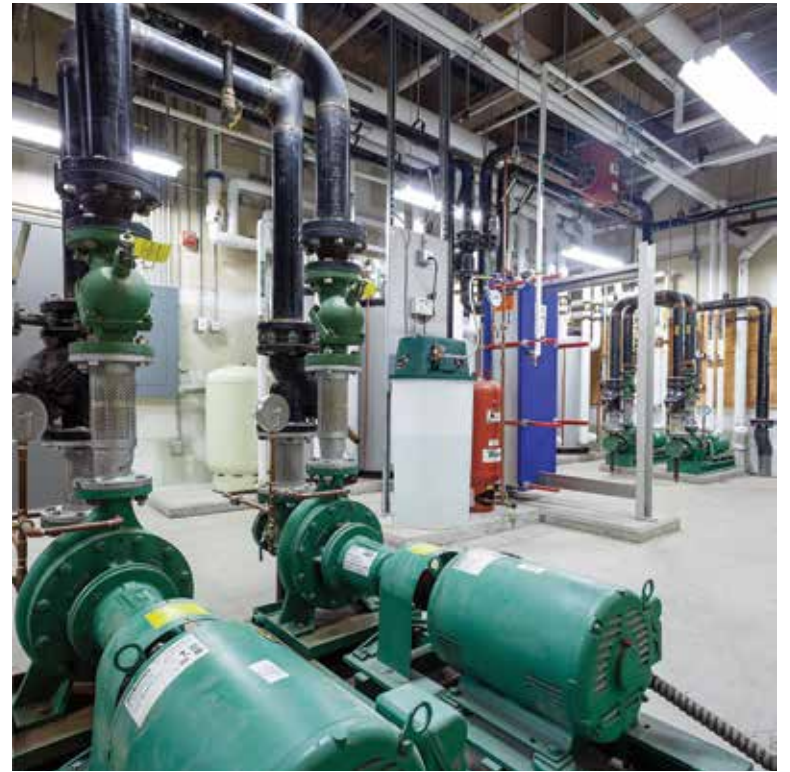
At Redstone Lofts, the south building’s mechanical room includes Taco FI Series loop water system pumps, the glycol reserve tank and its expansion tank, the large plate and frame heat exchanger, and cooling loop tower pumps.
