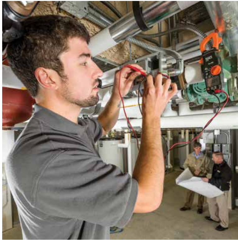
Matt Blair, Redstone Lofts maintenance manager, tests the variable frequency drive for Taco circulators that serve remote hydronic zones. The apartment complexes have been rated very highly by University of Vermont students.
