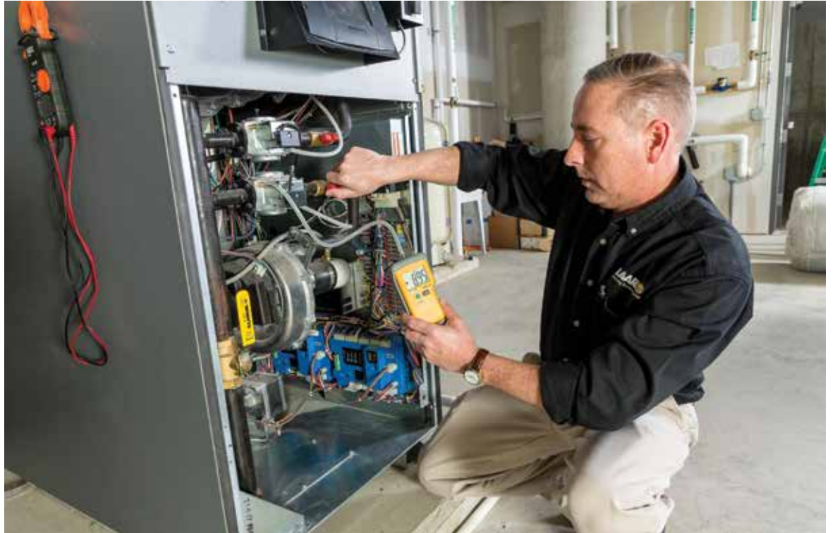
Steve Moruzzi, Laars territory service manager, tests the operating efficiency of a Laars NeoTherm.
