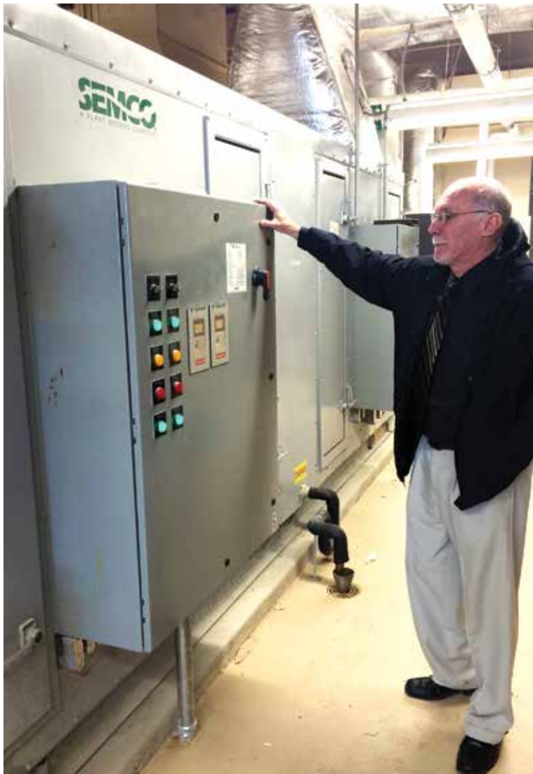
Paul Christy, superintendent, Clark County Public Schools, said the new high school’s dedicated outdoor air system (DOAS) and active chilled beams combination saved the district thousands of dollars within its first four months of operation.
