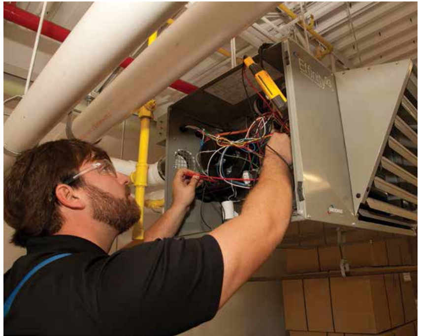
■ BIG OR SMALL: Proper venting for this small, Modine Effinity 93 unit heater is just as important as for larger systems.
