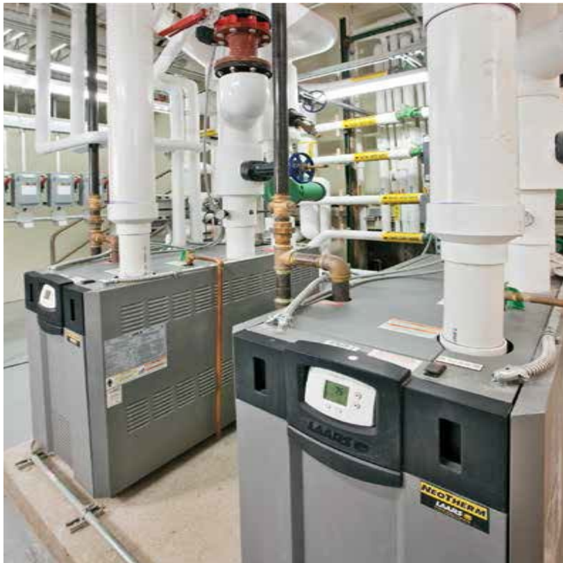
FUNCTIONALITY, ACCESSIBILITY: Venting becomes an important function and design element when laying out a mechanical room that assures not only proper function of all equipment, but easy access to all systems.
