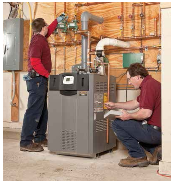
■ MAKING A LIST: As technicians button-up a completed light commercial hydronic system, satisfactory venting is on the checklist.
