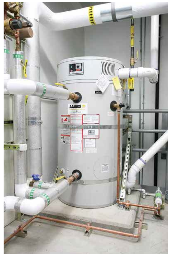
ALASKAN AD'VENT'URE: Proper venting for this high-efficiency Laars water heater was a key consideration by Weldin Construction pros when designing this mechanical space on a military base in Alaska.
